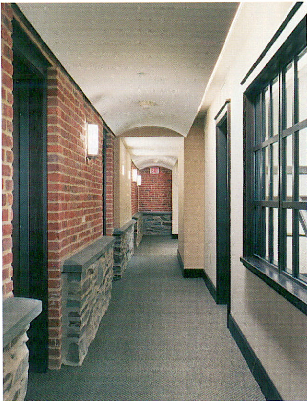
The foundation stone — as well as the brickwork — was all cleaned, repaired and repointed.
